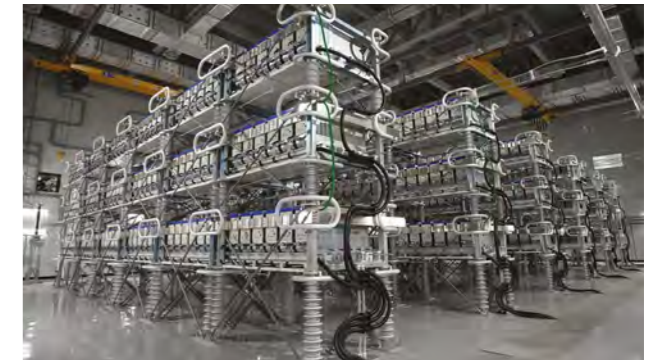
Figure 4 | Yangju Converter Valve
