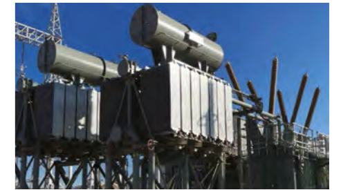
Figure 10 | Phase Shifting Transformer 330kV
