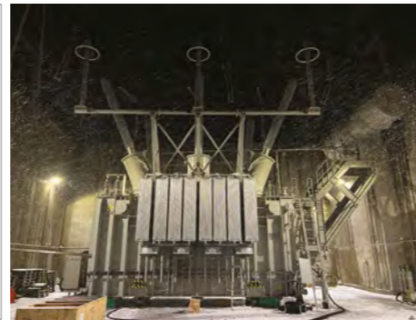
Figure 7 | Norway Auto Transformer
