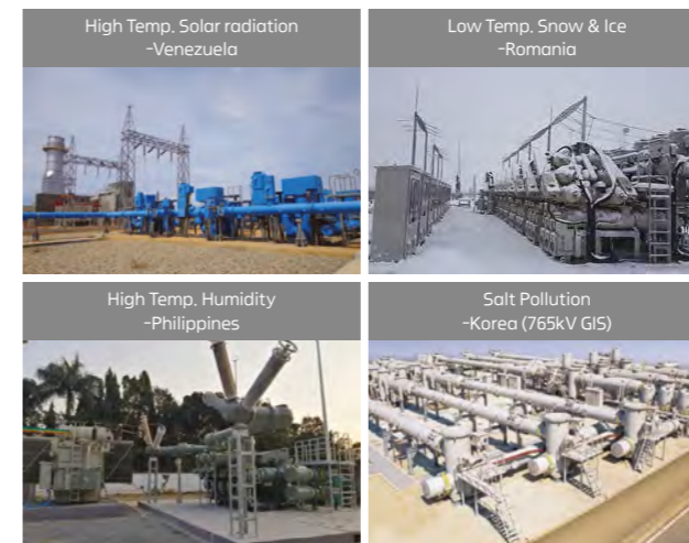
Figure 2 | Key Achievements of Hyosung Heavy Industries' Outdoor GIS
