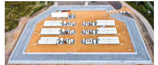
Figure 6 | BESS System Installed in South Africa
