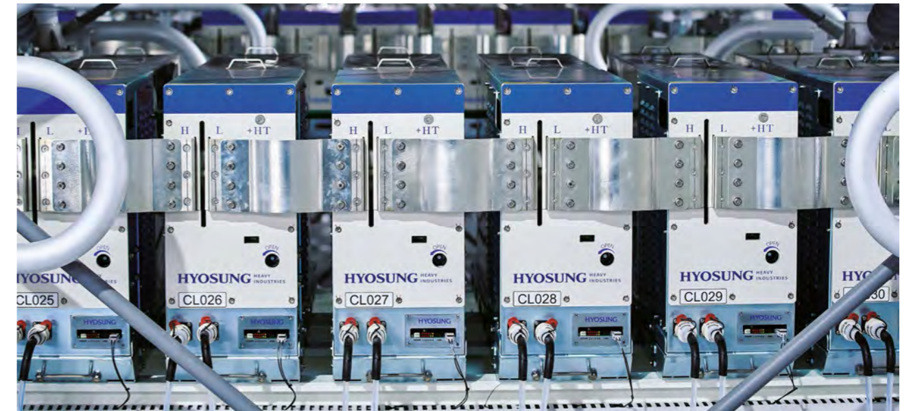
Figure 6 | A close-up view of Yangju converter valve
